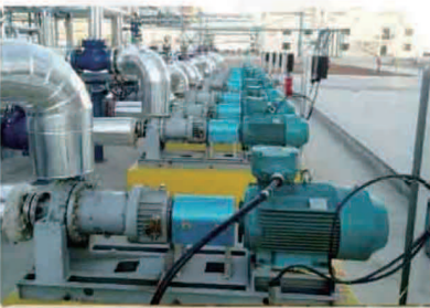
Chloride feed pump
