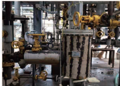
Liquid chlorine pump
