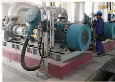
Chlorosilane feed pump
