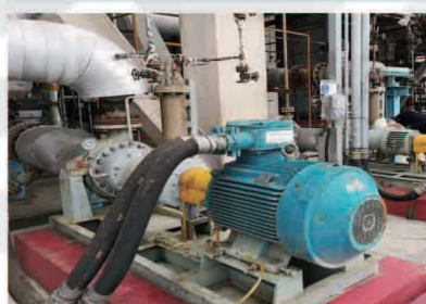
Quench tower circulating pump
